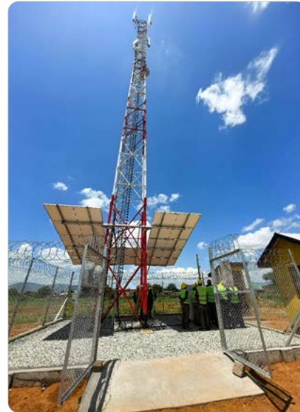
▲ Completed telecommunication site in Tanzania
