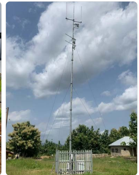
▲ Equipment in Ghana (telecommunication site)
